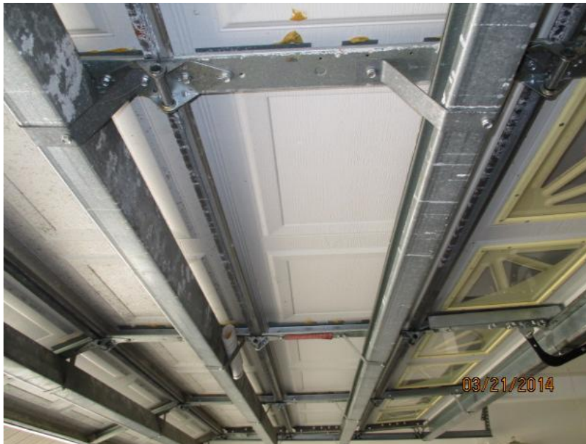
Unprotected Glazed Garage Door
