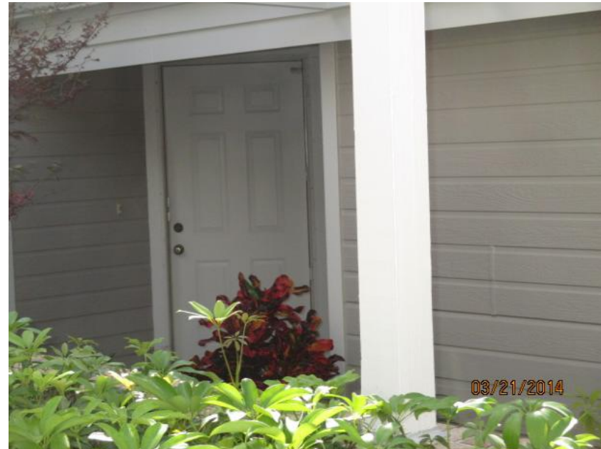
Unprotected Solid Entry Door
