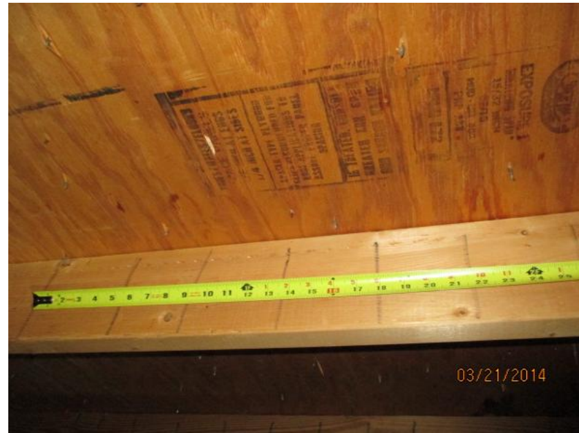
7d Nails Spaced 6" in the Field is equivalent to 8d nails spaced 12" in the field
