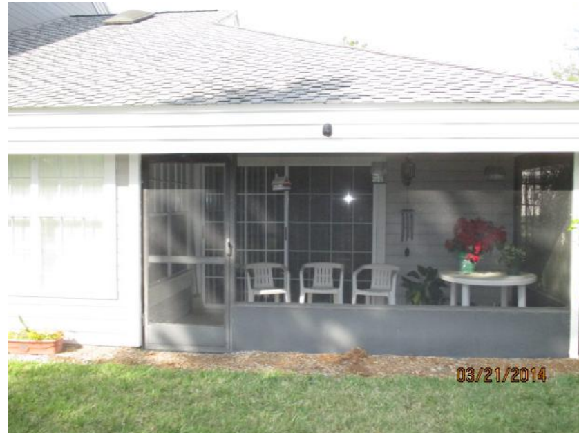
Unprotected Glazed Entry Door
