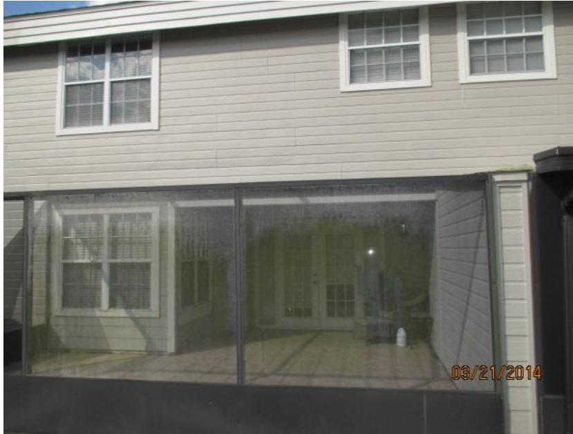
Unprotected Glazed Entry Doors
