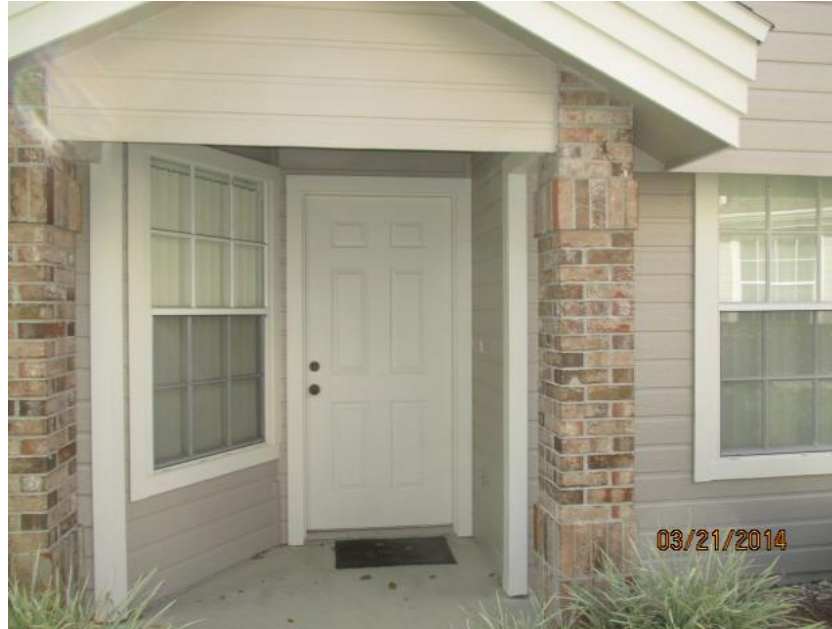
Unprotected Solid Entry Door
