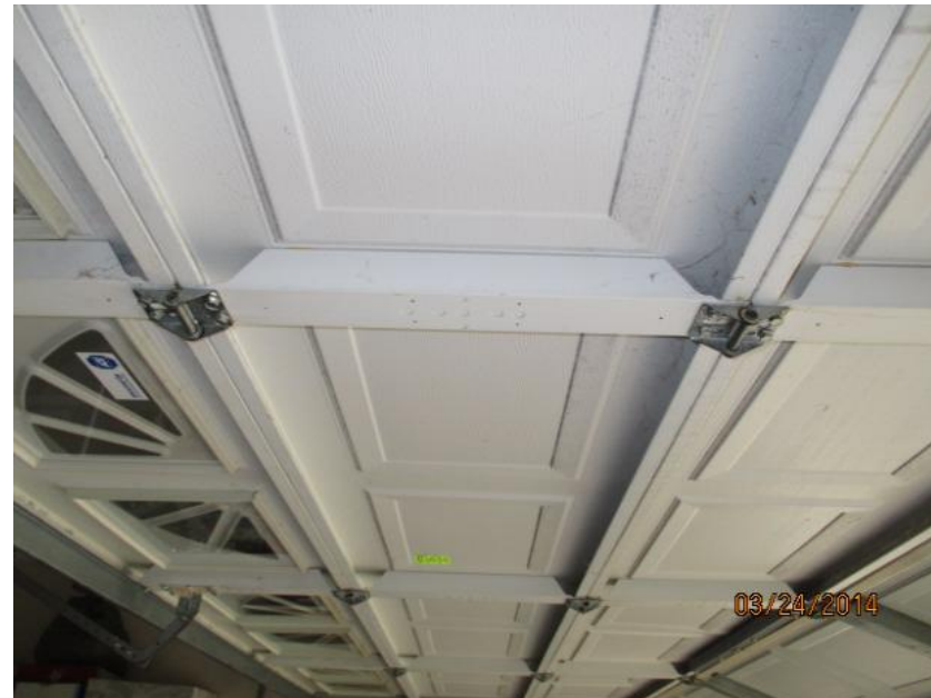
Unprotected Glazed Garage Door
