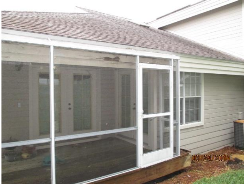
Unprotected Glazed Entry Doors
