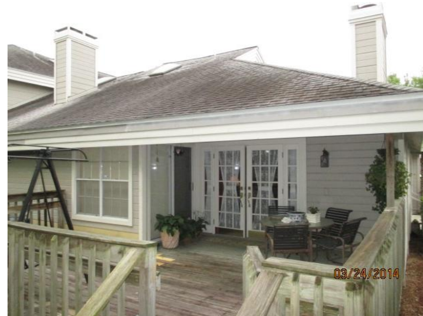
Unprotected Glazed Entry Doors
