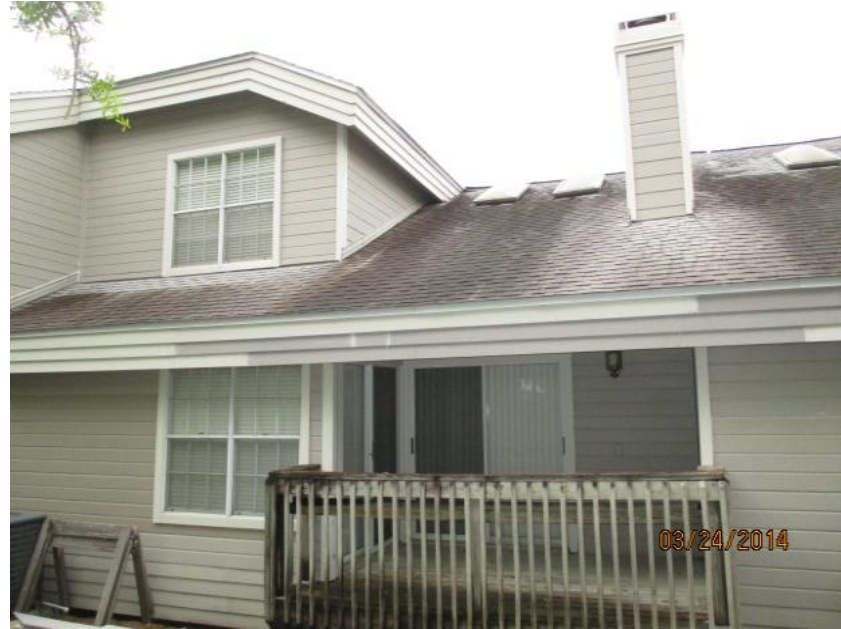
Unprotected Glazed Entry Doors
