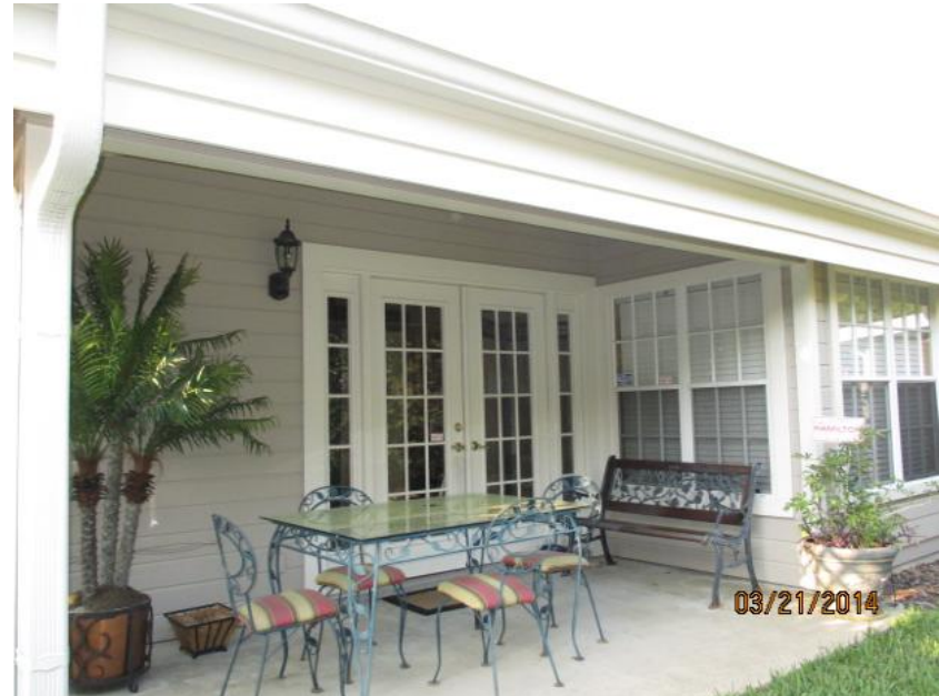
Unprotected Glazed Entry Doors
