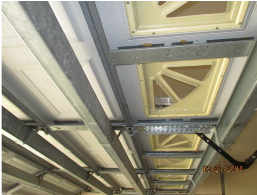
Unprotected Glazed Garage Door
