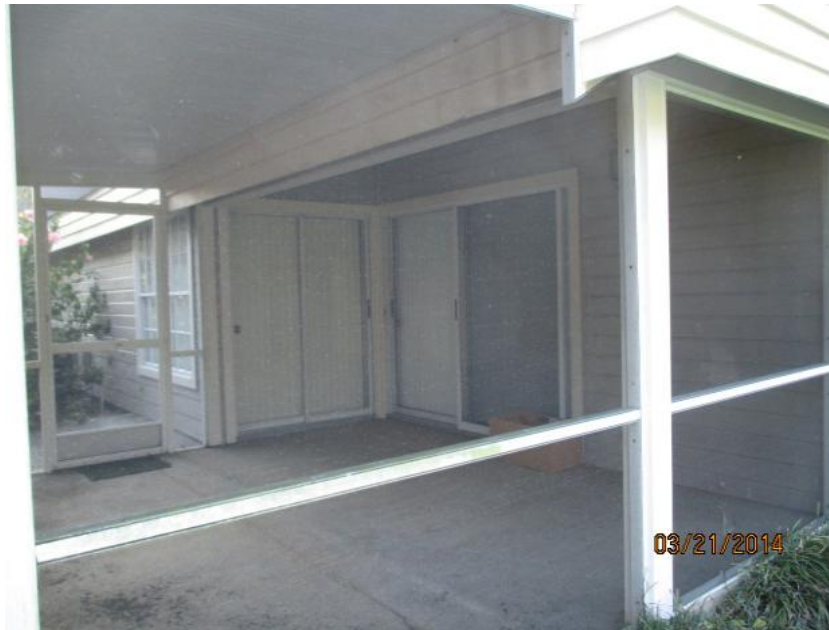
Unprotected Glazed Entry Doors
