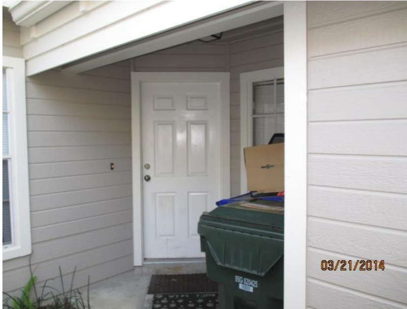
Unprotected Solid Entry Door
