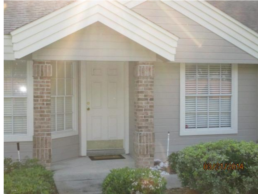
Unprotected Solid Entry Door
