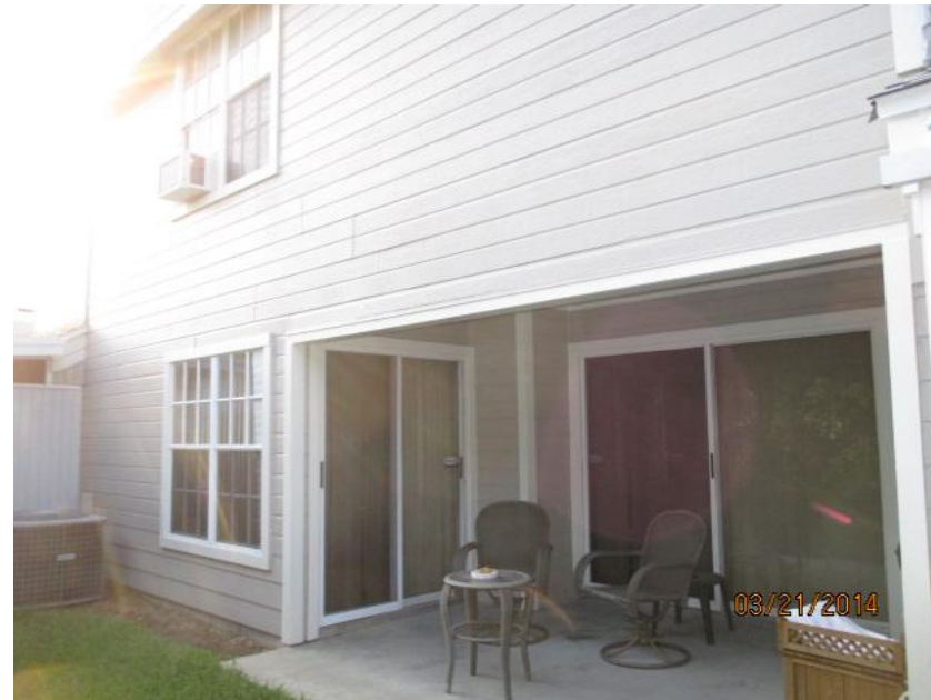
Unprotected Glazed Entry Doors
