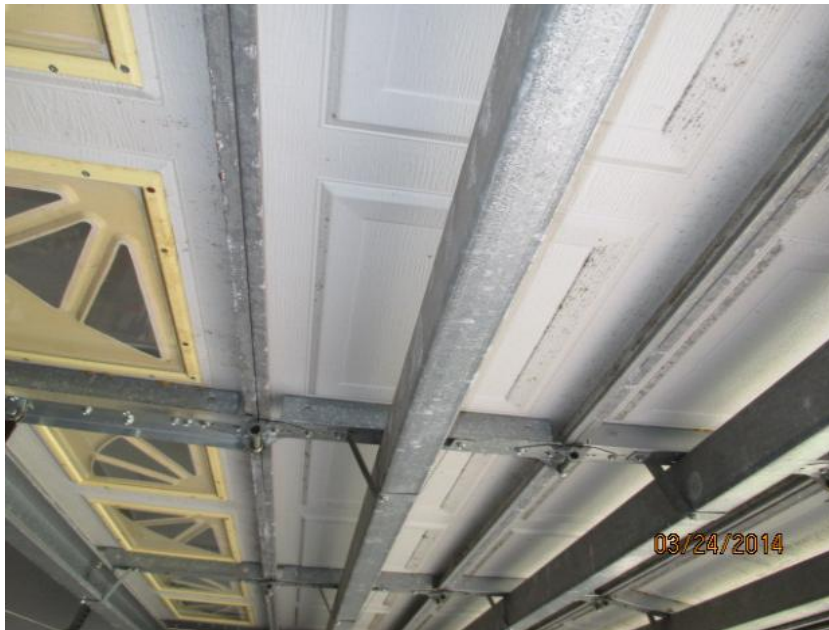
Unprotected Glazed Garage Door
