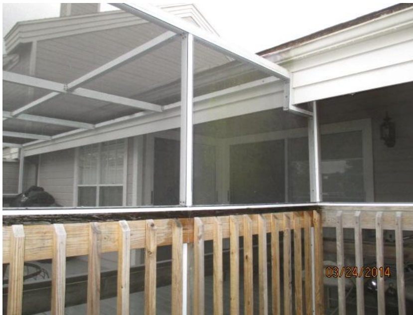
Unprotected Glazed Entry Door
