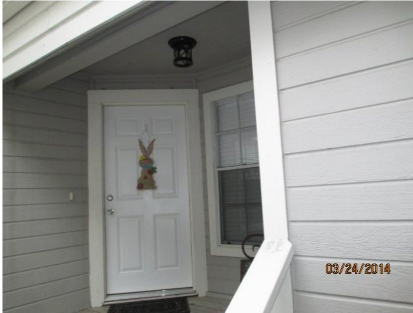
Unprotected Solid Entry Door
