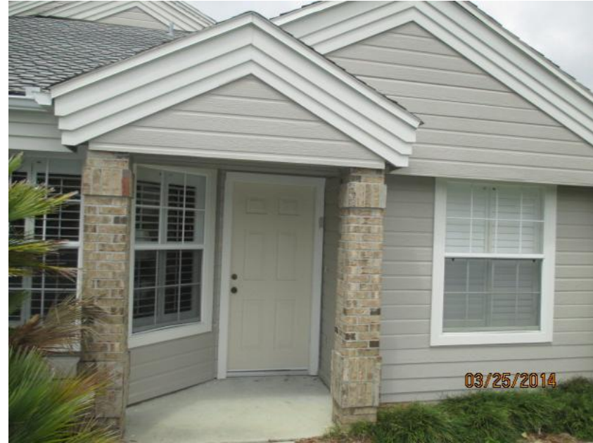
Unprotected Solid Entry Door
