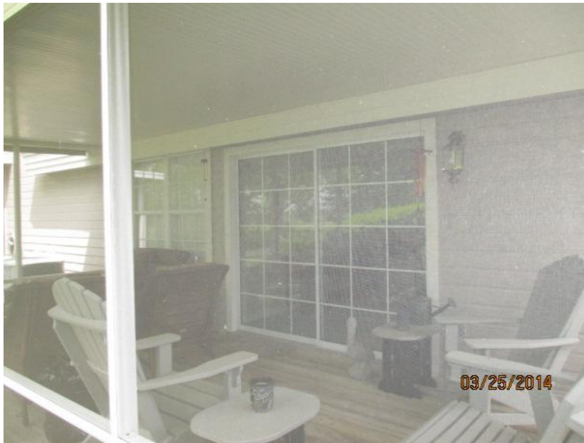
Unprotected Glazed Entry Door
