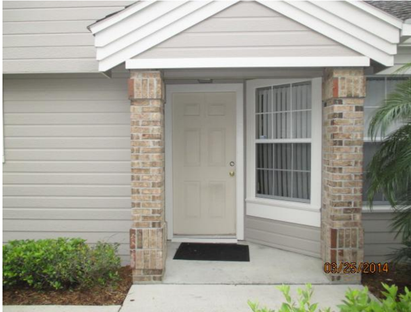
Unprotected Solid Entry Door
