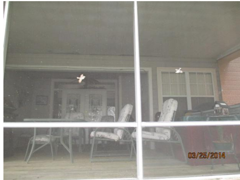
Unprotected Glazed Entry Doors
