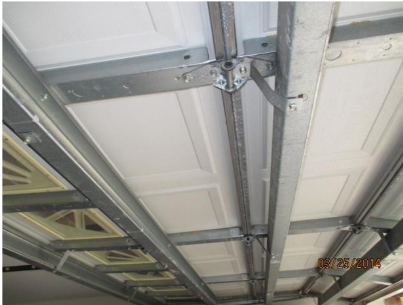
Unprotected Glazed Garage Door
