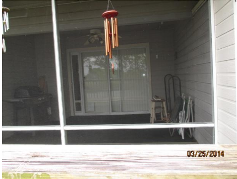
Unprotected Glazed Entry Door
