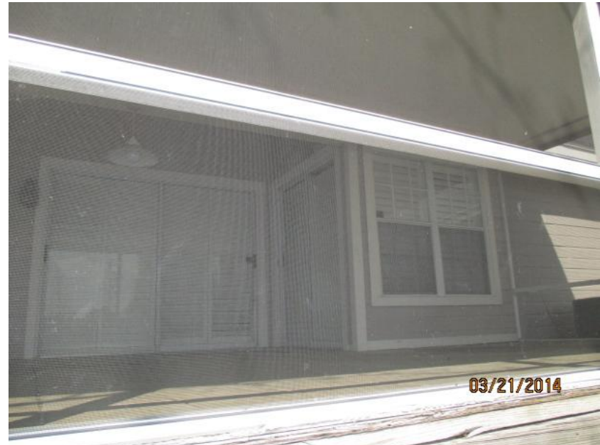
Unprotected Glazed Entry Door
