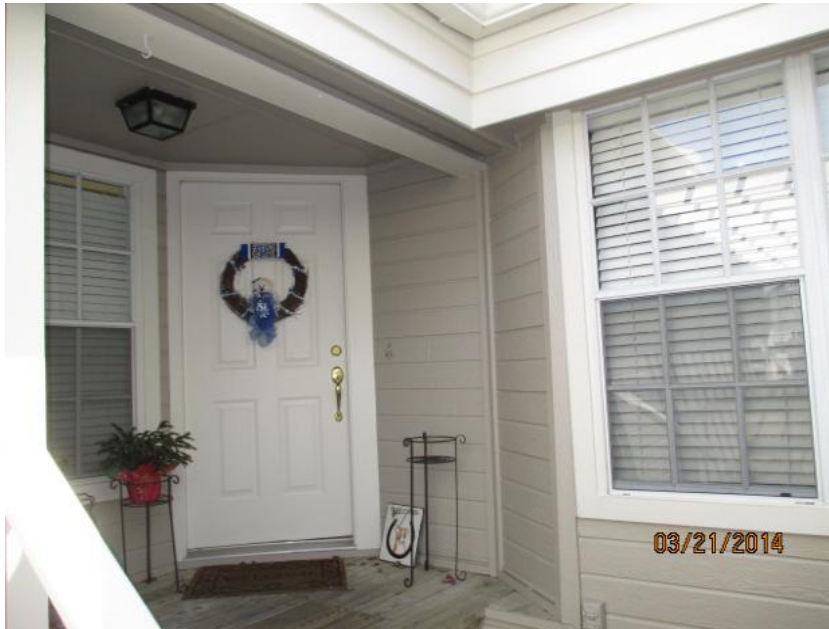
Unprotected Solid Entry Door
