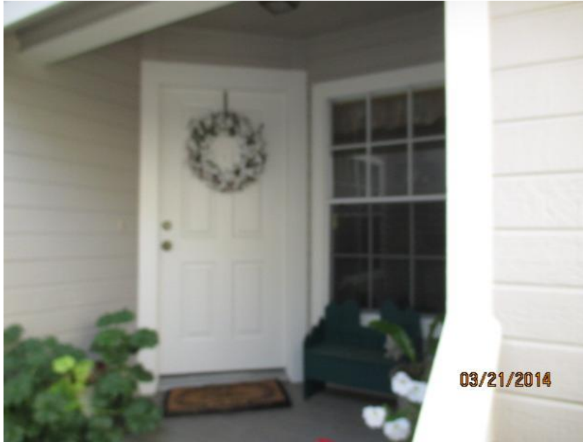
Unprotected Solid Entry Door
