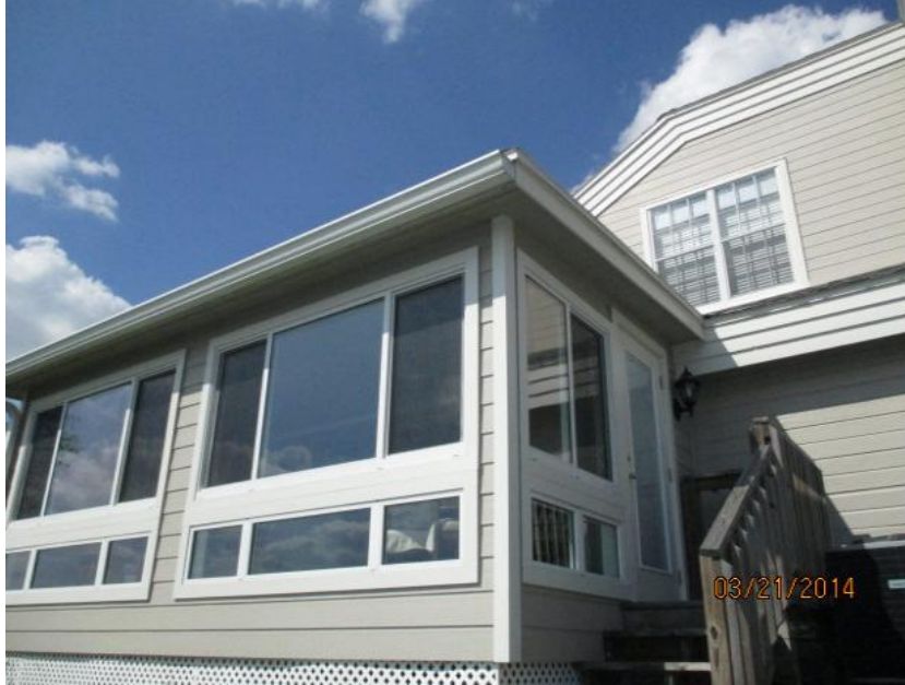
Unprotected Glazed Entry Door/ Windows
