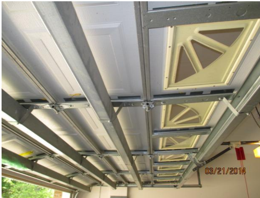
Unprotected Glazed Garage Door
