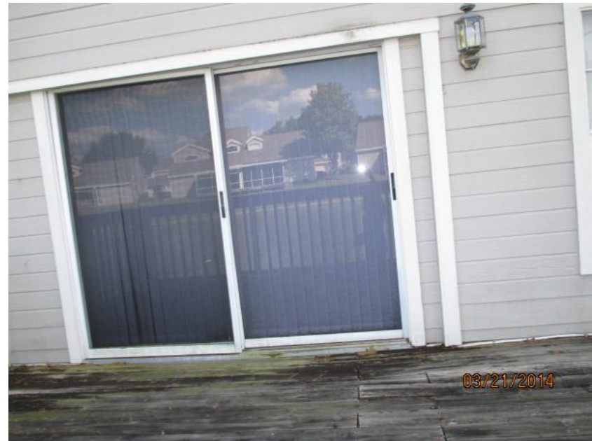
Unprotected Glazed Entry Door
