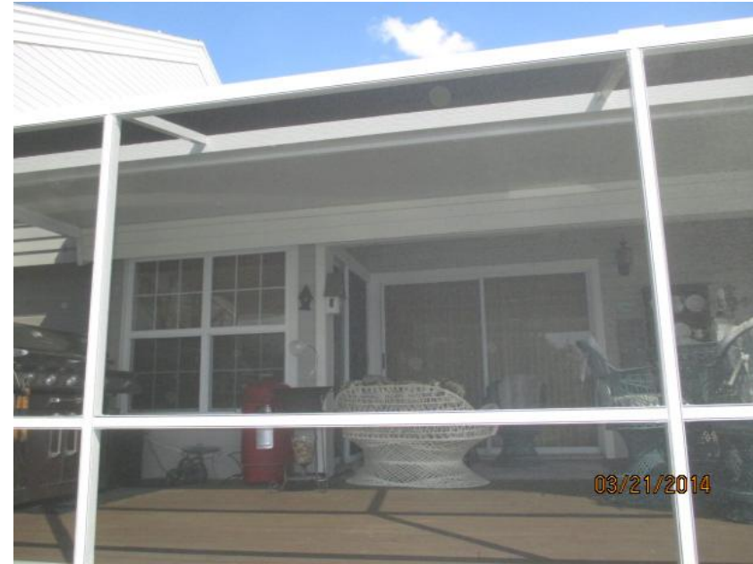
Unprotected Glazed Entry Doors
