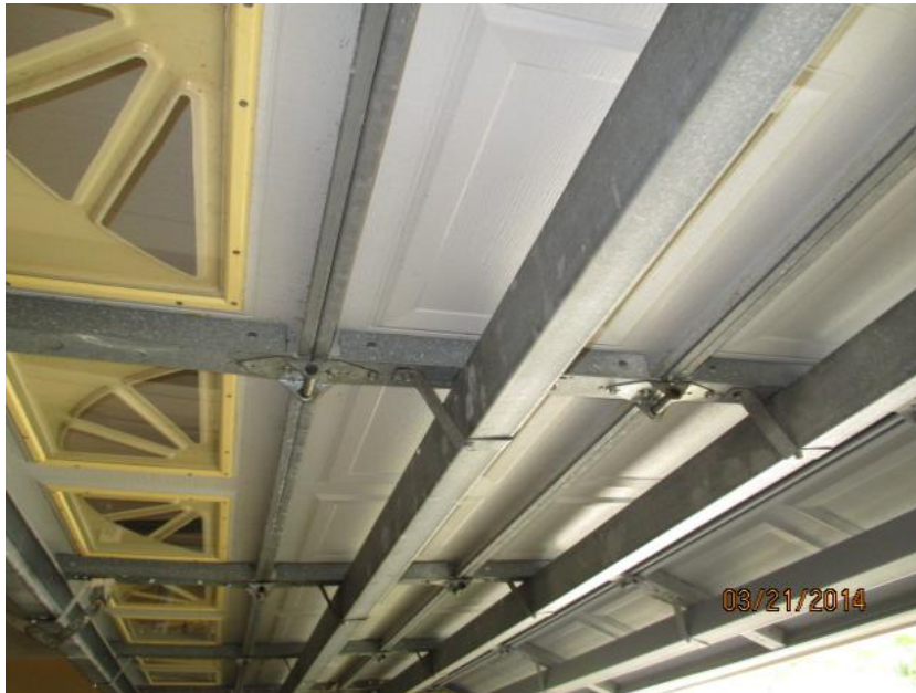
Unprotected Glazed Garage Door
